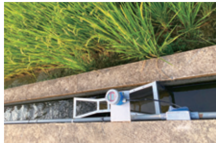
Parshall flume flow meters
