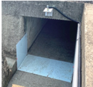
Ultrasonic water level sensor
